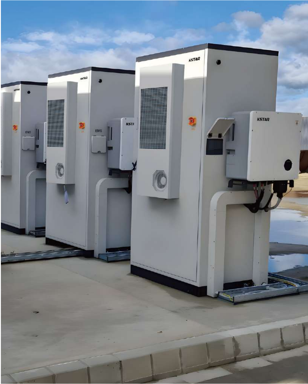
07 C&I ESS-project in Hongarije
