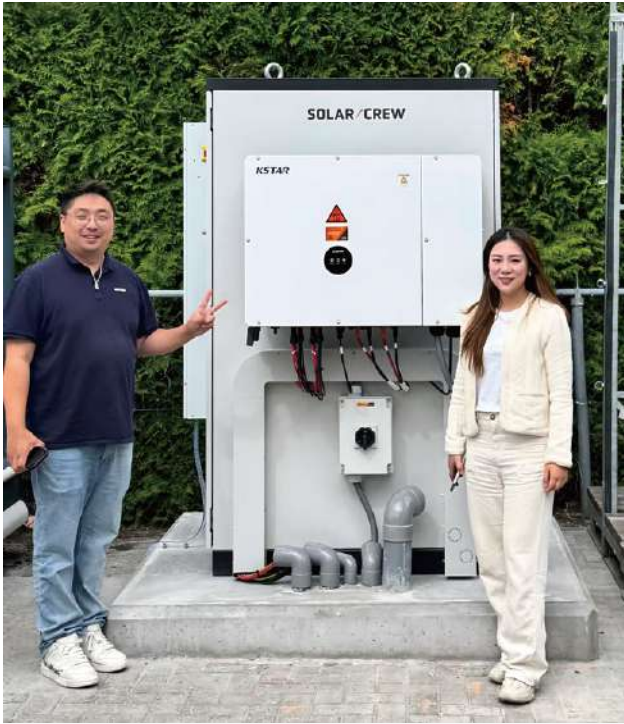
01 C&I ESS Project in Nederland
