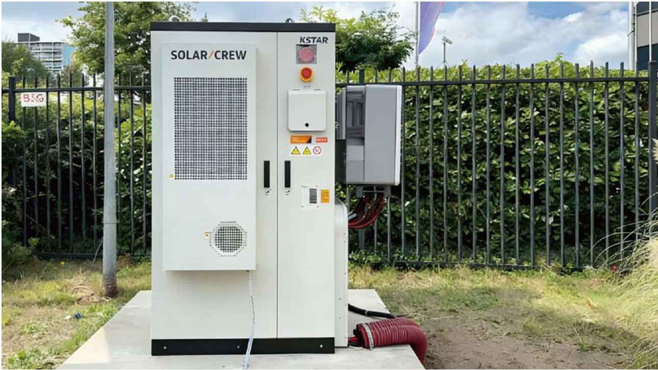
04 C&I ESS Project in Nederland
